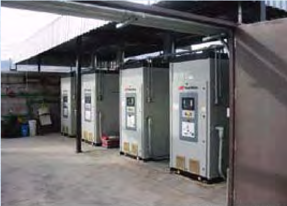
PHOTO: SCS ENGINEERS
