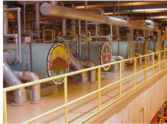
Boilers, located above the engines
