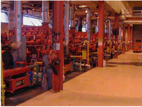
Seven 650-kW Waukesha engines
