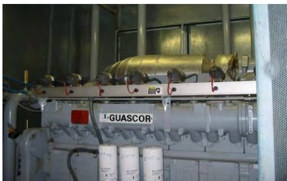
290-kW engine retrofitted to run on biogas, from Belgium-based Continental Energy Systems
