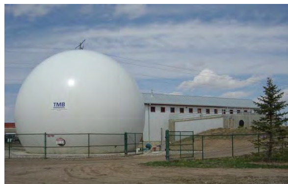
New Belgium Brewery's 225,000 gallons/day process water treatment plant with anaerobic and aerobic digestion
